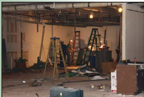
Renovation of the Davidson Family Health Sciences Building which will house the F. Marie Hall SimLife Center at Midland College began in Summer 2011. Completion is expected in December.
